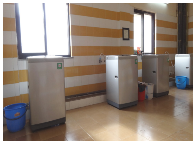
The new washing machines installed in HR4
