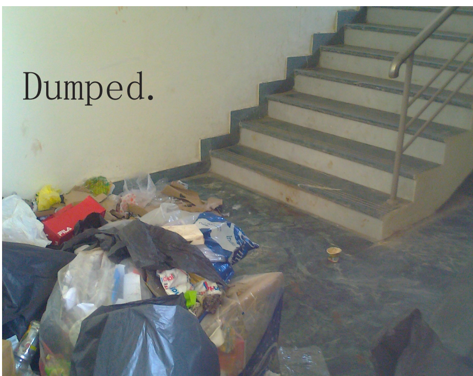
Heaps of garbage dumped on the stairway in the new hostel
