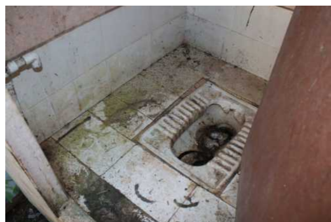
Bathrooms and toilets used by the workers living behind the girls' hostel
